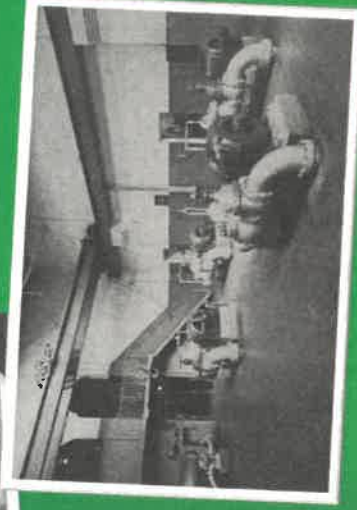
Water processing pumps
