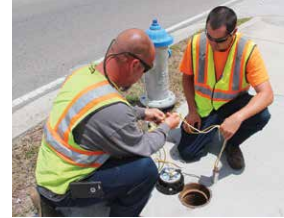
James White (left) and John O'Dell, Water Technicians, deploy electronic sound detectors within water infrastructure.
