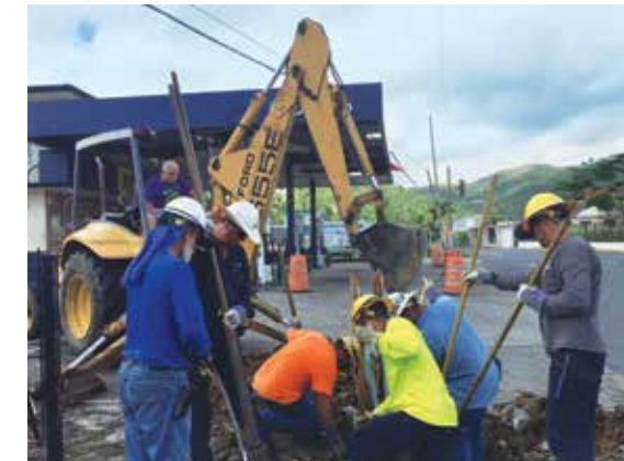
OUC crew members Luis Burgos, Bryan Walsh, John Wallace, Andre Phillips, Mike Atout and Chris Trainiello work to remove the base of a broken pole along the transmission line from the Rio Blanco Hydroelectric Plant to the Juncos Substation on PR 31, a major highway between the towns of Naguabo and Juncos in Puerto Rico.
