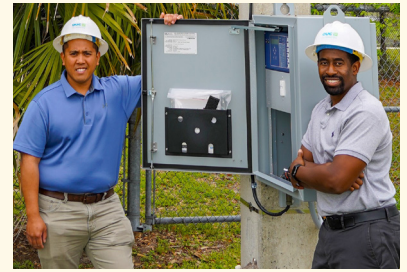
Steve Casios (left), Sr. Distribution Engineer, and Fabian Richards, Manager of Distribution Planning and Reliability Engineering, check a FLISR control unit installation.
