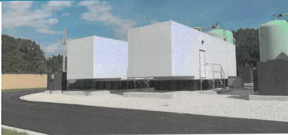
* Emergency Gen Sets Conway
